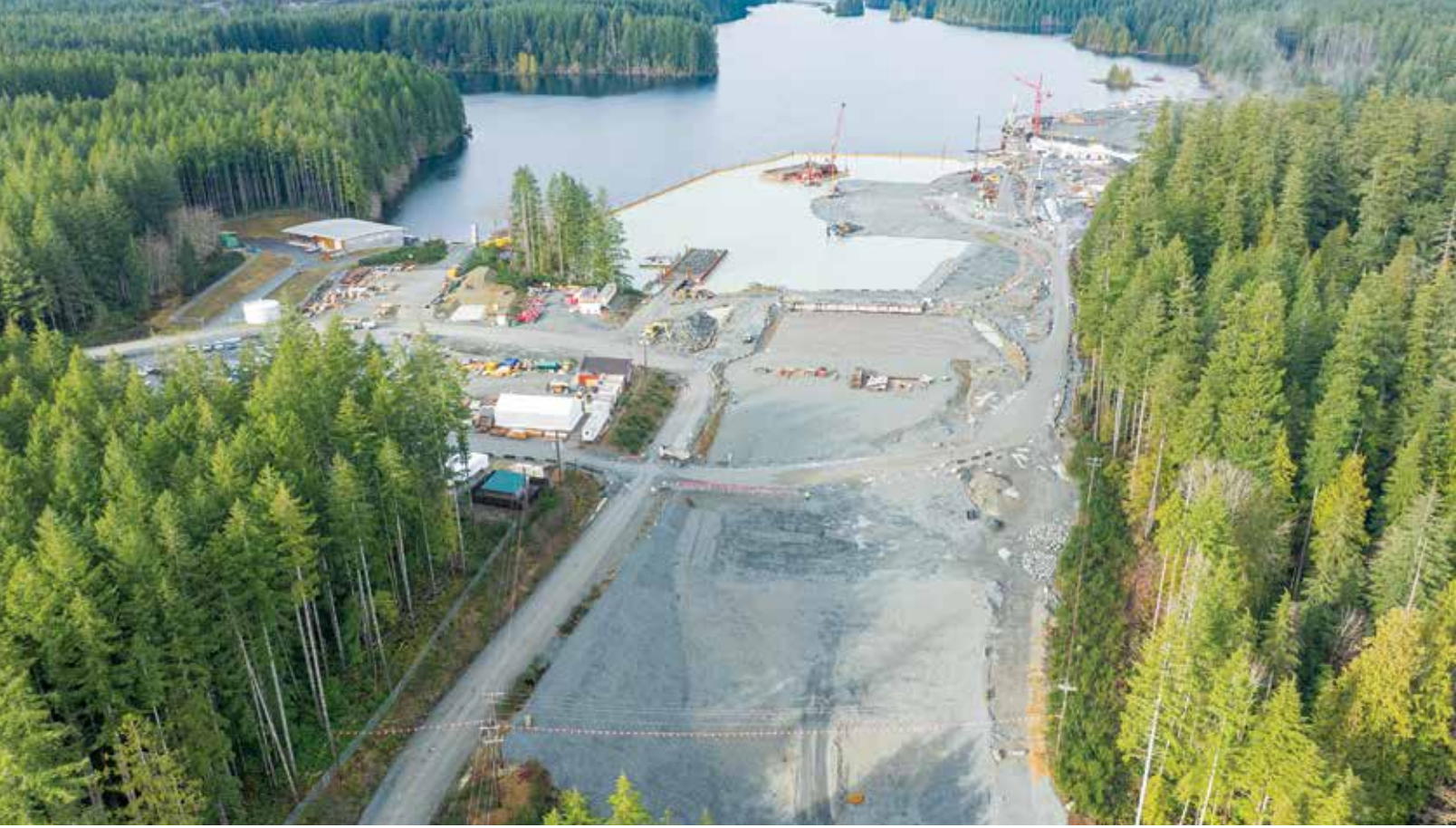
Rock placement work around the Old Intake Dam within the John Hart Reservoir. PHOTOS COURTESY OF BC HYDRO.
