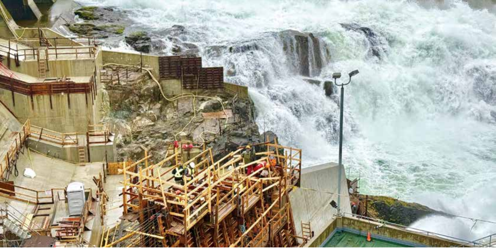
Work on the downstream concrete works at the base of the new overflow spillway.
