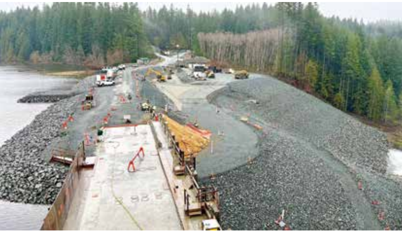
View of the dam and the new berms from the spillway gates.
