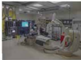
Diagnostic Imaging Installations
