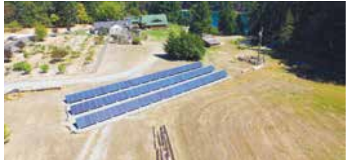
This 26-kilowatt solar system built by Osprey Electric on Gabriola Island, B.C., is one of the largest residential solar system installations in the province.
