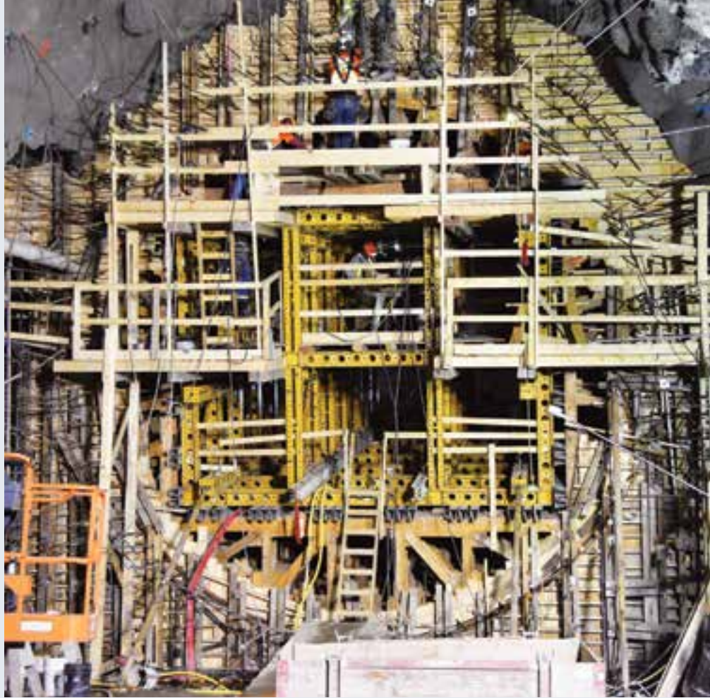
The power tunnel manifold located just before the powerhouse area is approximately 8.5 metres in diameter.
