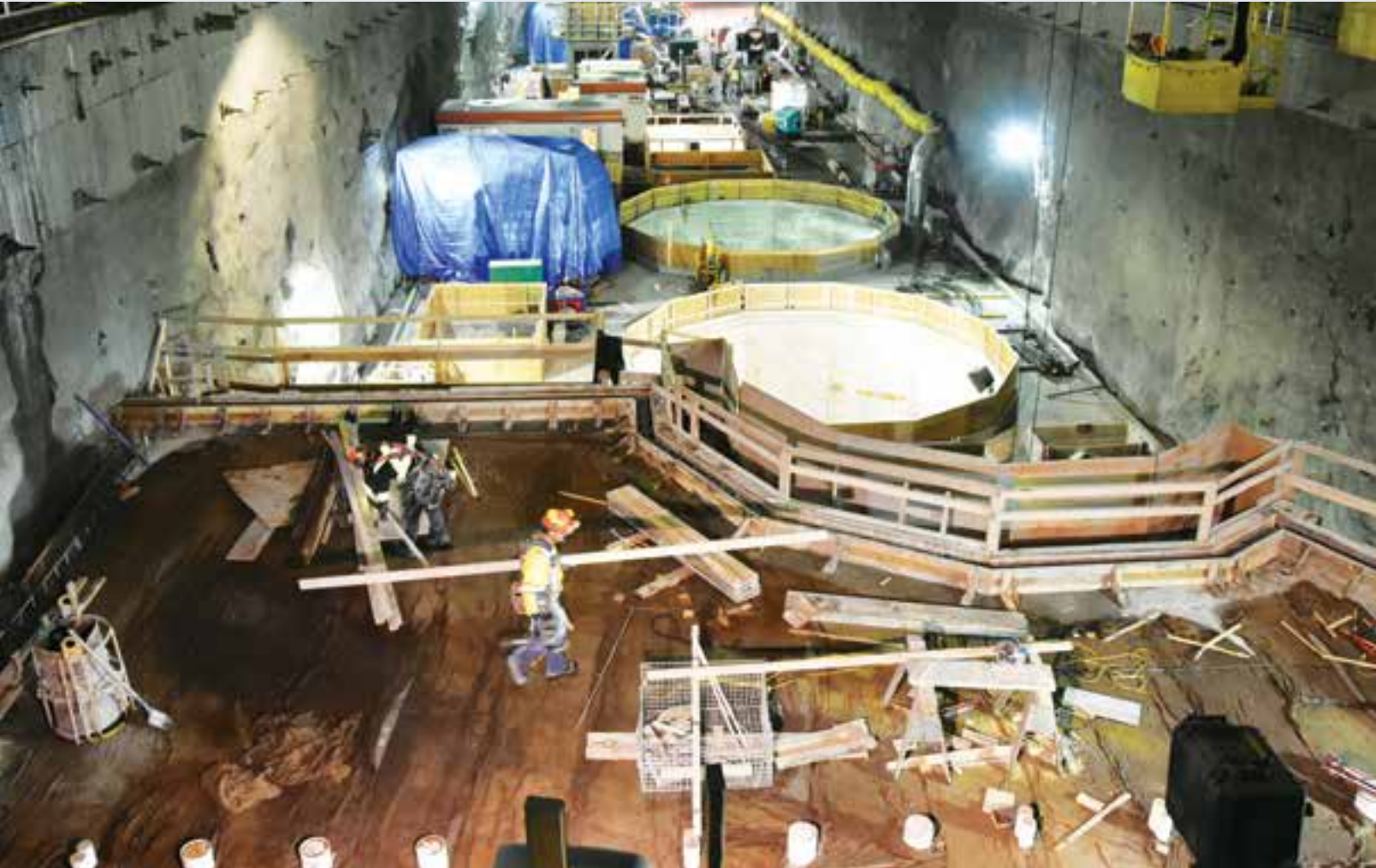
Powerhouse cavern – the underground powerhouse is 10 stories high and as long as an NFL football field.
