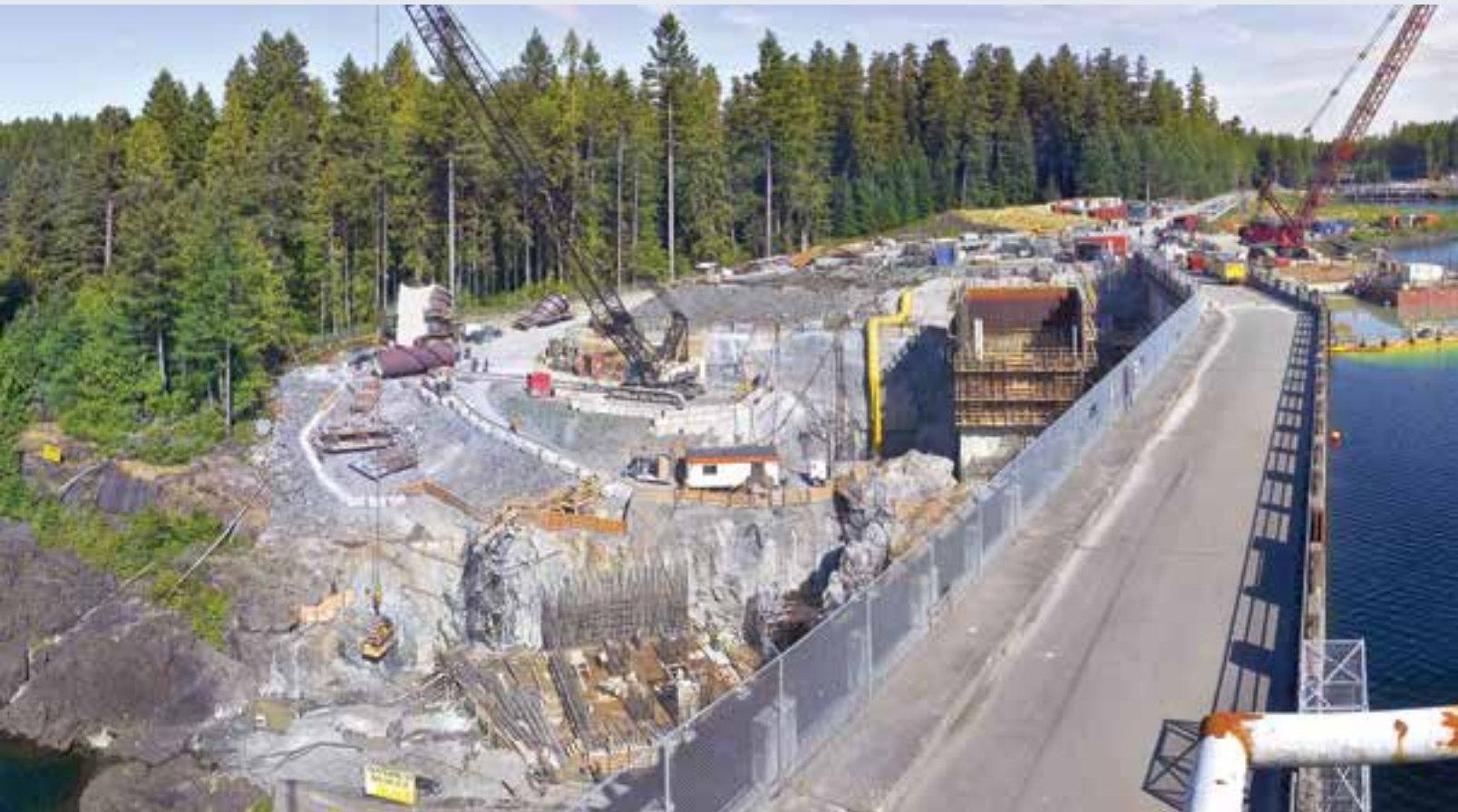
New water intake works at the John Hart dam where water will enter the power tunnel and travel about 1.6 km to the underground powerhouse.
