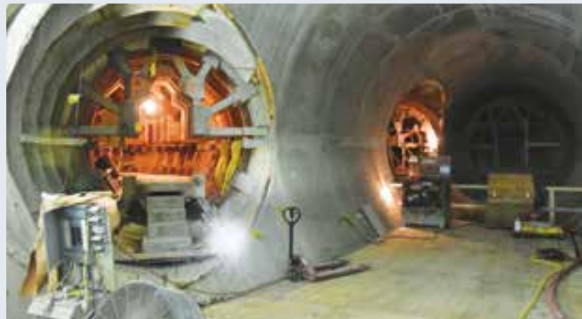
View inside the power tunnel manifold and the water inlets to the three turbines/generators taken December 11, 2017.
