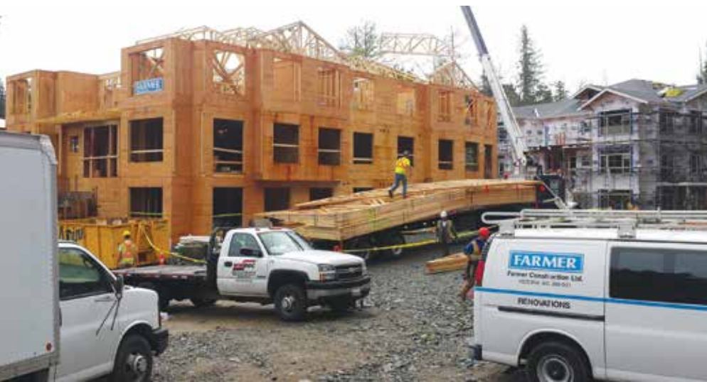
Rain screen going up on Building #3, while trusses are lifted onto Building #4.
