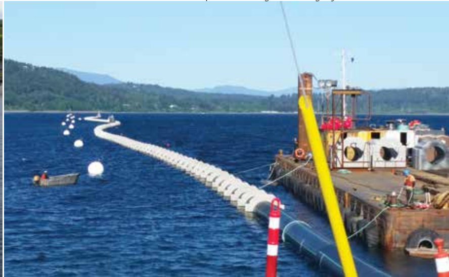
Assembled precast weight units surround the completed pipe section prior to moving and sinking in final location.
