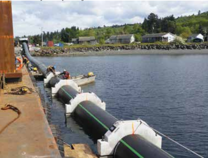
Completed precast weight units being numbered and labeled for ease of locating once under water.
